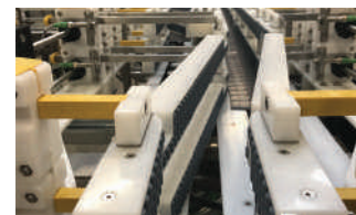
Automated Conveyor Y gate.
